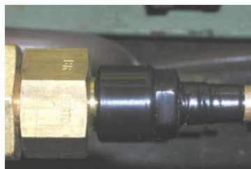
Photo 2 Mounted union Doubly protected
